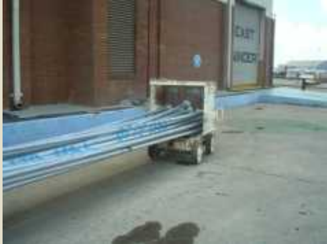
Wrong bogey used
